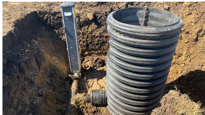
Figure 3. Gate Structures to Control Water Table
